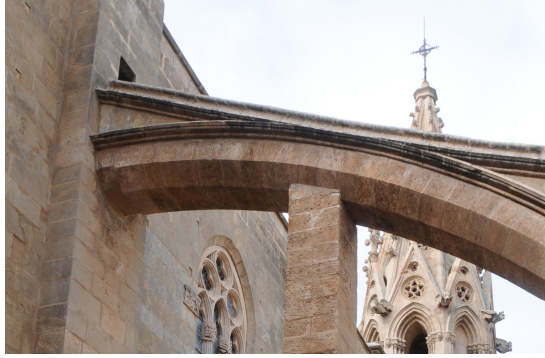
Figure 14. Sliding in the upper flying buttress B6N. Note that the sliding is not between the wall and the first voussoir, but between first and second voussoirs [Photo: Roland Wiczorek, BTU Cottbus-Senftenberg].
